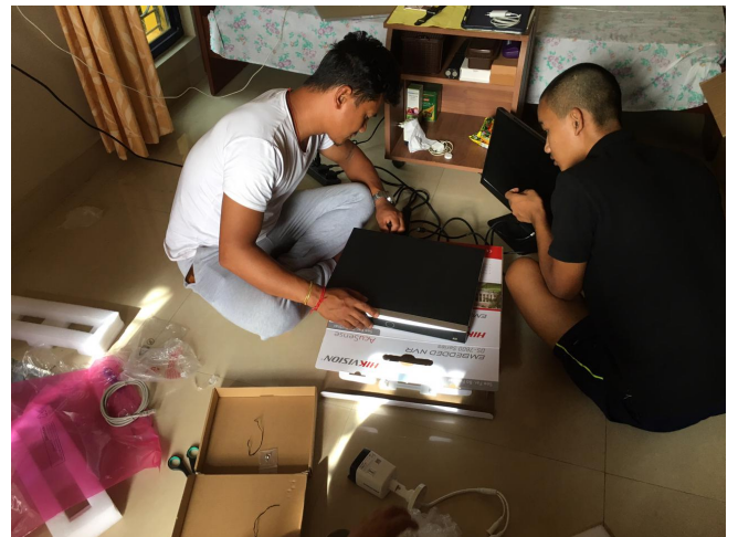
H. Installation of CCTV's in the property of the ACT, 29th April, 2023.
