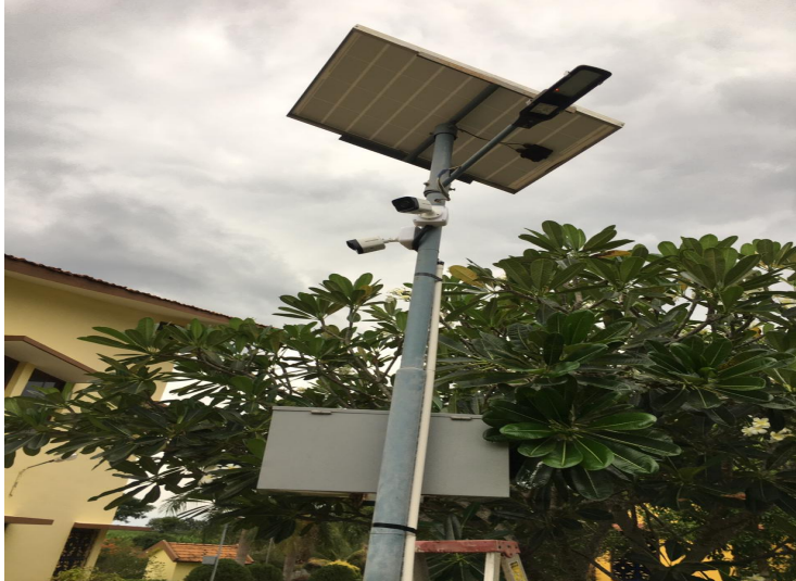
H. A view of the CCTV Cameras, 29th April, 2023.
